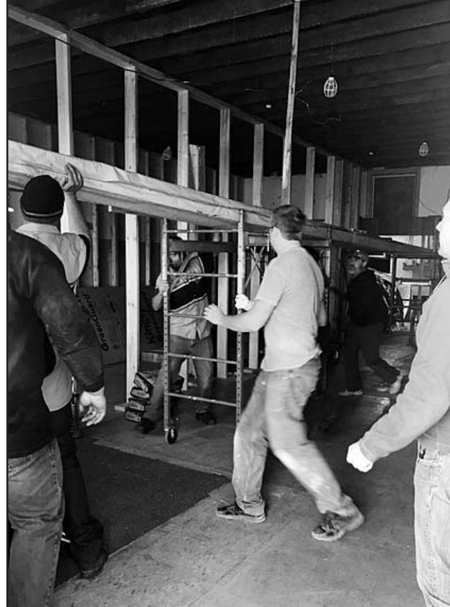
Inside the building, the beam is guided onto scaffolding by Larreau Construction's crew and the volunteers. Pictured in the center of the room is a temporary wall that was built to hold the sagging roof after it was jacked up about 6 inches to level.
