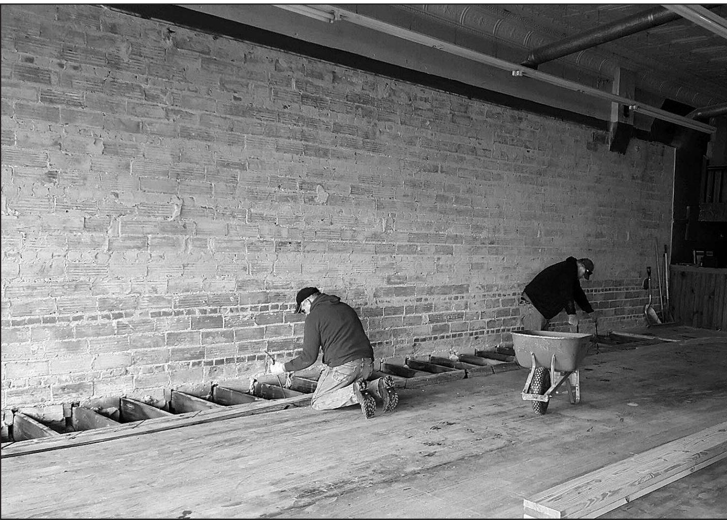
Keith Knight and Greg Tickle work on the floor joists of the 1914 building that will be the future home of BrewBakers Coffee House and Gifts on Arnold's main street. In view are the original tin ceilings, brick walls and wood floors that have been uncovered. (Courtesy photo)
