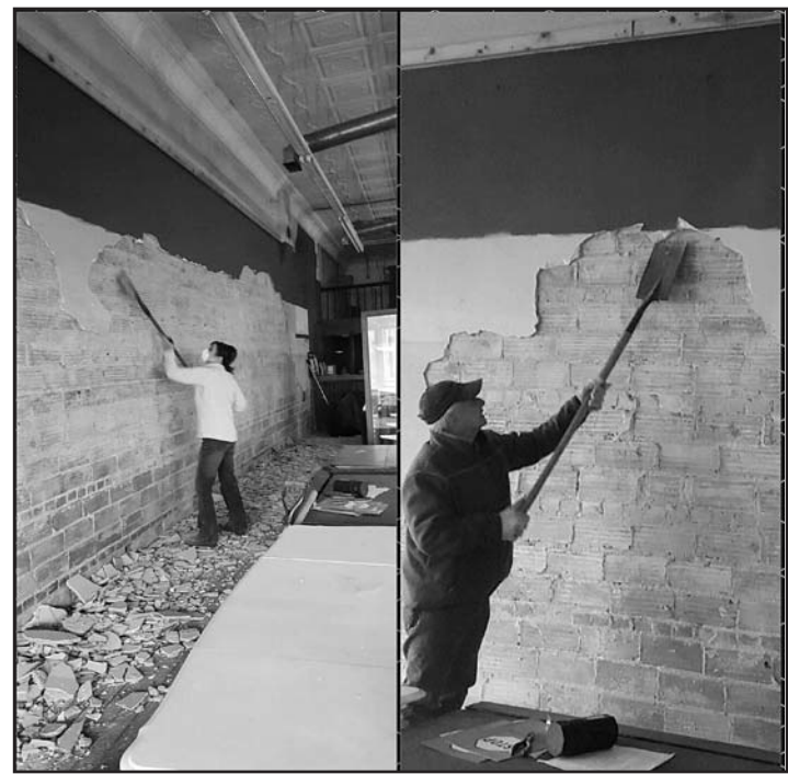
Jodi Carlson (left) and Keith Carlson (right) work to expose the original brick walls of the building.
